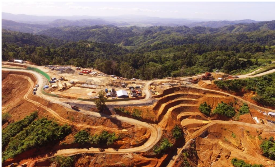
Aerial view of Mill Plant Site of the Balabag Gold Project at January 27, 2020.
